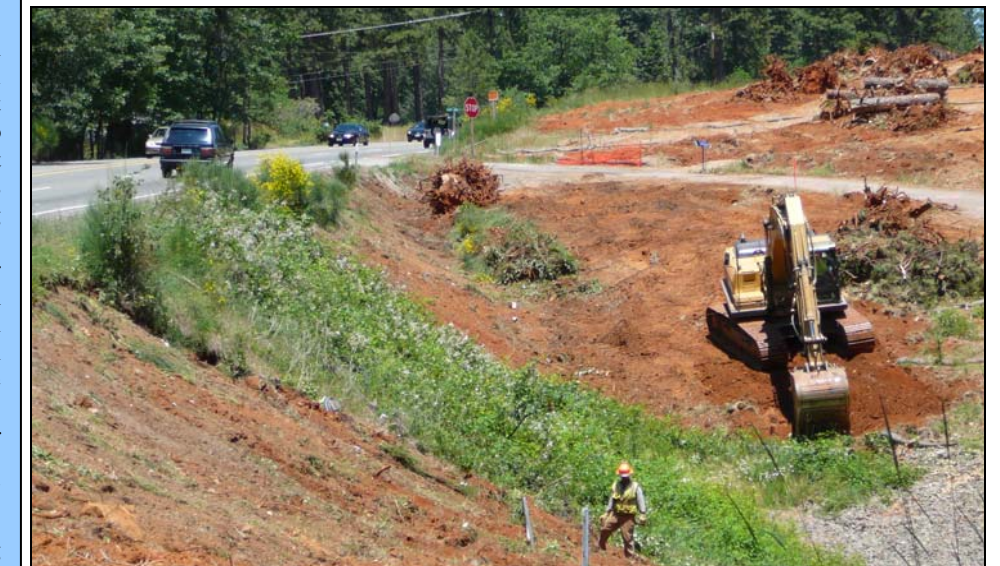
Crews clear tree stumps before constructing frontage road on east side of SR 49
