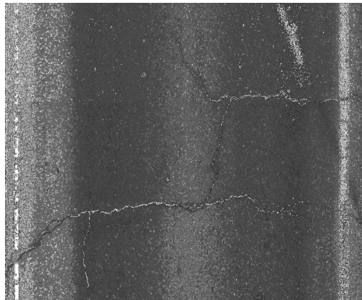
Example of High Definition Cracking Image
