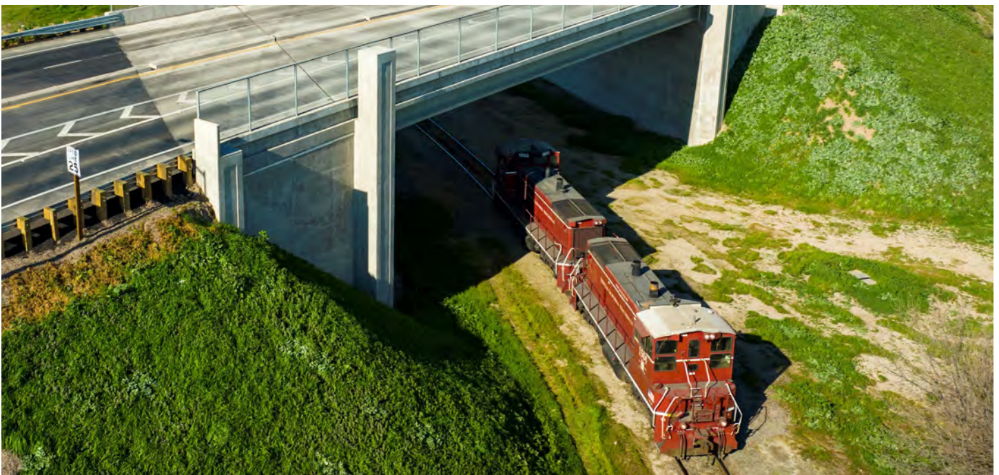
Funded through the Trade Corridor Enhancement Program, the Fyffe Avenue Grade Separation project constructed a four-lane overcrossing over the Fyffe Avenue rail line and removed an at-grade intersection. This project reduces travel times for vehicles entering the Port of Stockton, thereby facilitating the movement of goods. Removing the at-grade intersection also provides vehicle and rail safety improvements and enables a critical emergency evacuation route.
